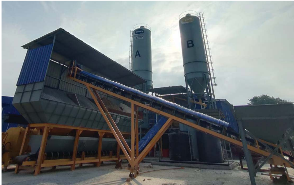
One of our concrete batching plants
