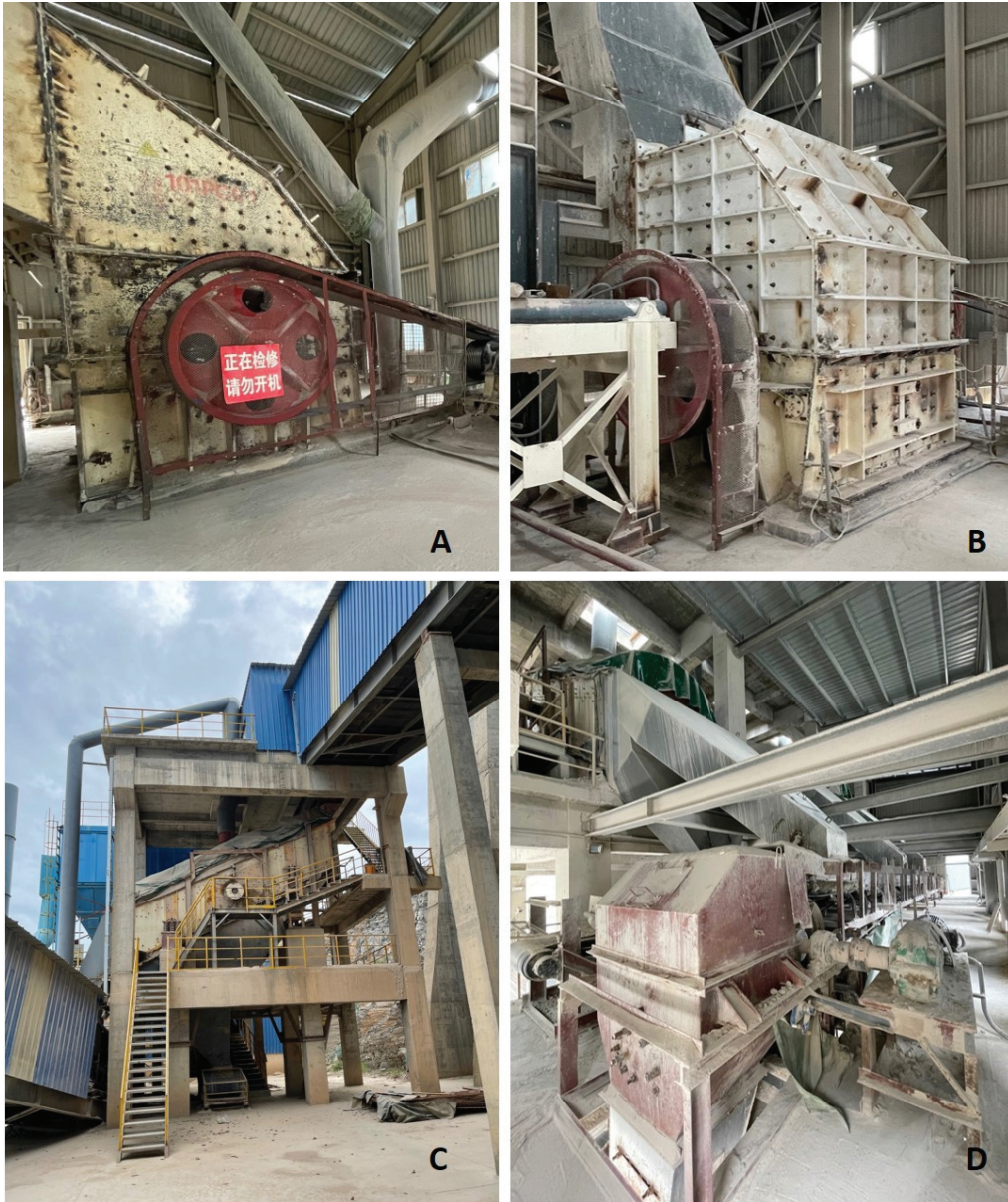
Figure 8-3: Phase I processing plant
