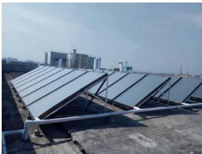
Solar heating system of Jiangmen Factory
