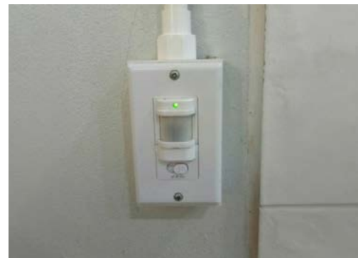
Installed light motion sensors to lower electricity consumption when rooms or operation area is not frequent use.
