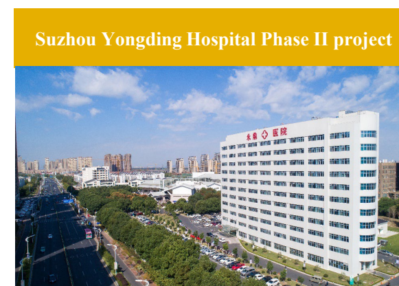
The preparation works of the Suzhou Yongding Hospital Phase II project has commenced Expected to additionally accommodate approximately 500 beds when it commences operations
