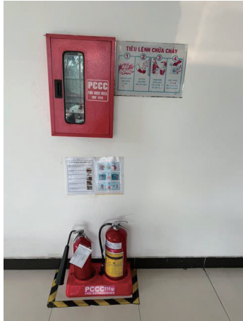
The fire protection equipment in factory area
