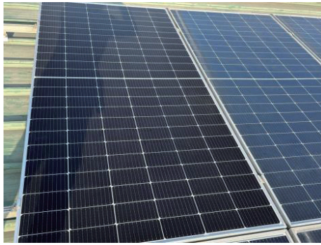
New solar PV panel installed in Vietnam factory
