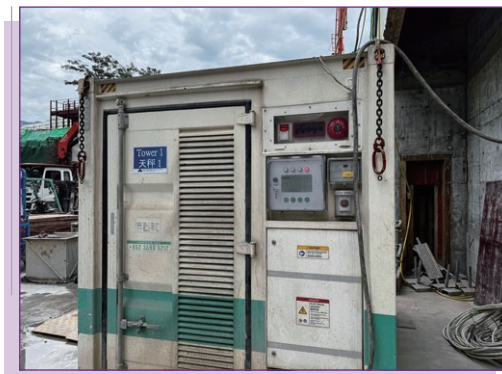
Innovative energy storage in our sites 於我們地盤的創新儲能
