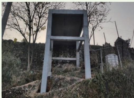
Completion of the construction of main body of the Convenience Pavilion in Daxin village, Rongshui county
