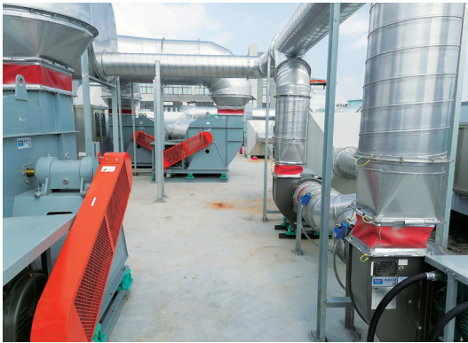
Upgraded Emissions Treatment Facilities 升級後的廢棄處理設施
