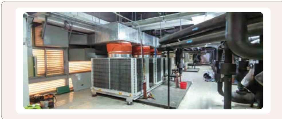
Air-cooling unit 1 repairing in the Onward Science & Trade Centre, and the renovation of the cooling tower in the HP Building 招商局航華科貿中心進行1號風冷機組更換與惠普大廈冷卻塔更新改造
