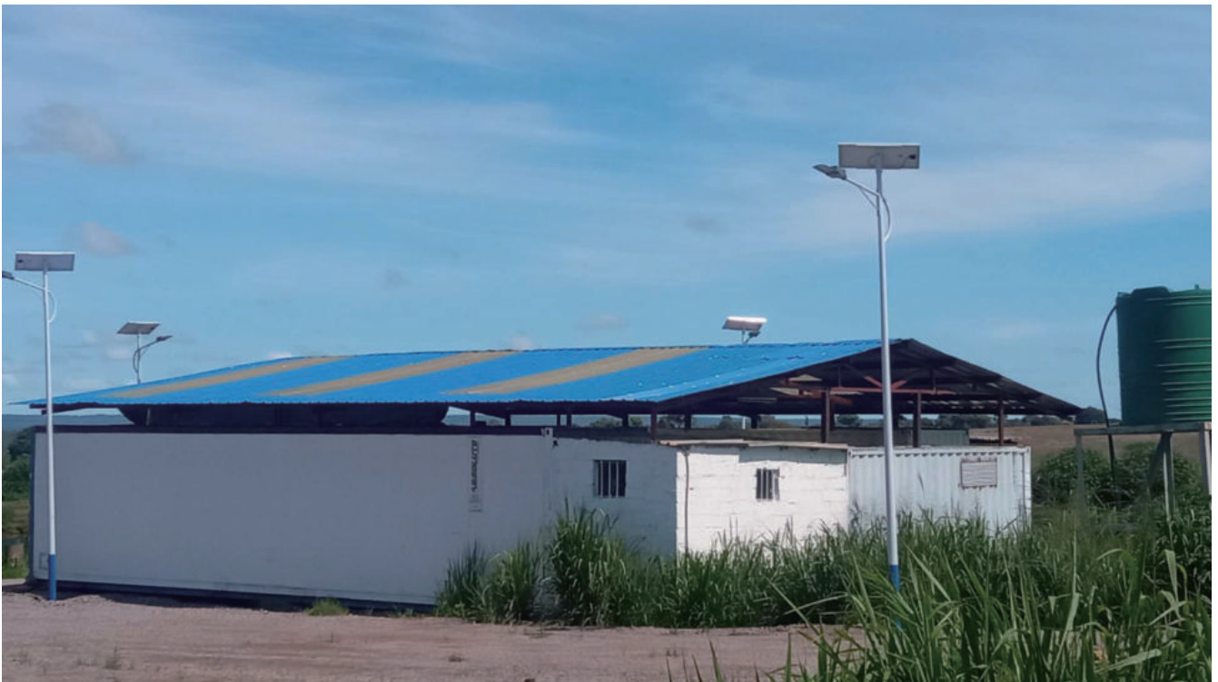
Kinsenda礦場太陽能路燈 Kinsenda Mine Solar Streetlights
