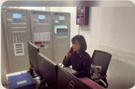
Real-time communications with surveillance operators
