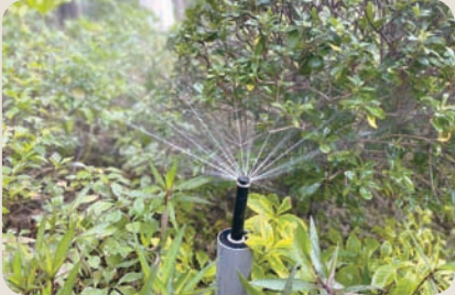
Automatic Sprinkler System
