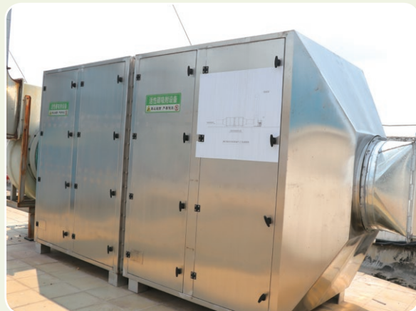
After the renovation of the printing treatment exhaust gas system 印刷處理廢氣系統改造後
