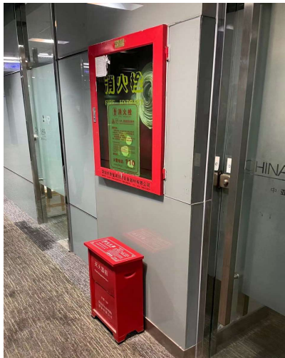
Fire safety equipment installed in the service site in Shenzhen
