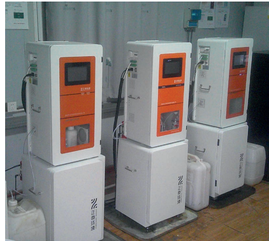
污水檢查設備 Sewage inspection equipment
