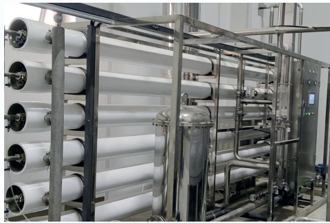
蚌埠鮮食廠反滲透處理設備 Reverse osmosis treatment equipment in Bengbu fresh food factory
