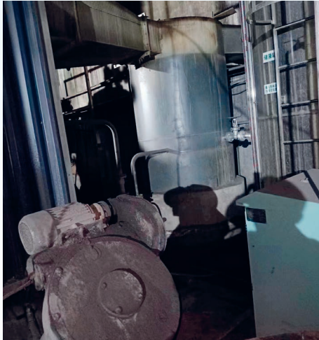
大連美食廠鍋爐安裝碳鋼無縫管配套節能器 A carbon steel seamless tube matching energy-saving device is installed on the Dalian food factory boiler
