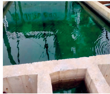
大連美食廠鍋爐軟化水處理 Boiler softened water treatment in Dalian food factory
