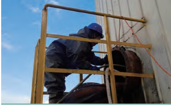
Shandong Linshu waste-to-energy project conducted equipment maintenance and safety inspection rectification actions 山東臨沭垃圾發電項目開展設備檢修及安全隱患排查整治行動
