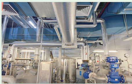
Steam pipeline insulation for energy conservation
