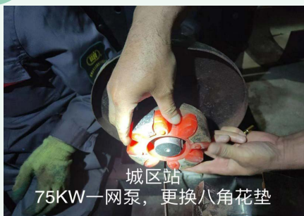
City Station 75KW circulation pump of a network, replace the aniseed cushion
