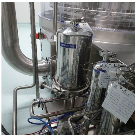
Recycled water filter of a bottle washing machine
