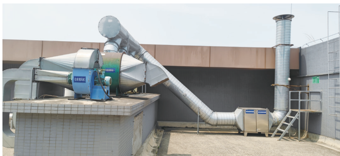
Waste disposal equipment
