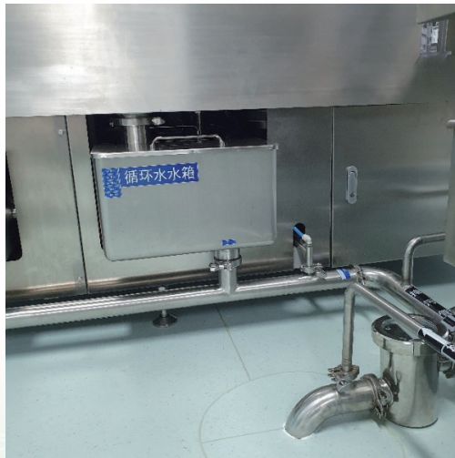
Recycled water tank of a bottle washing machine
