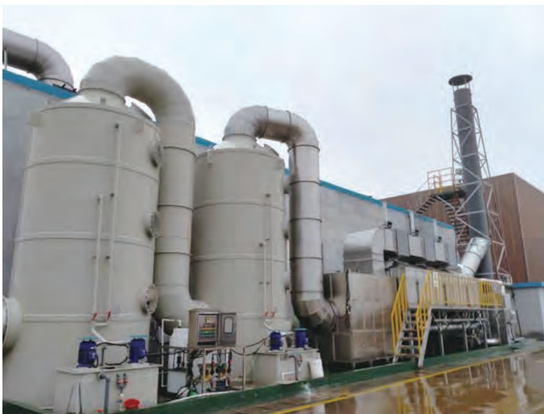
Figure 2 VOC treatment facility for reducing fugitive emissions at Xiangshui NU
