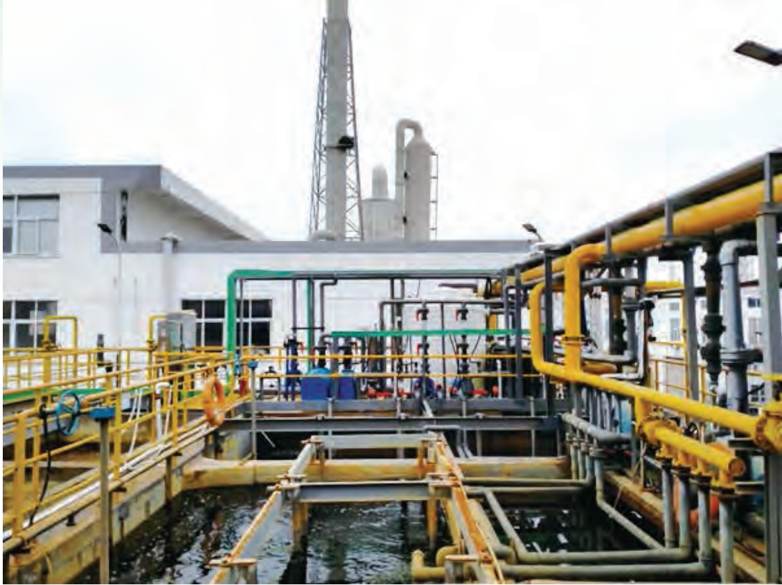
Figure 7 ROT-upgraded wastewater treatment facility at the Eco-Plating Specialised Zone
