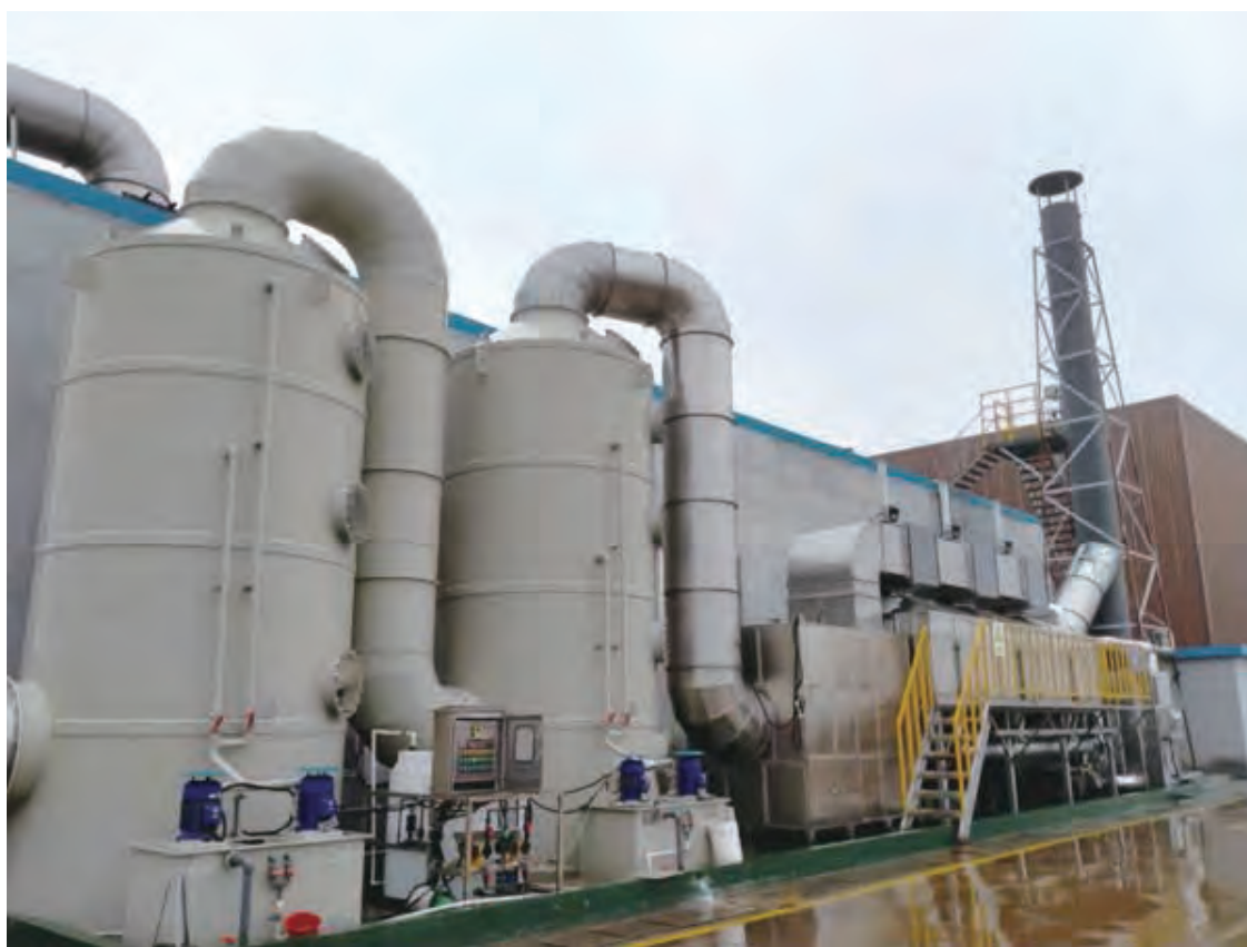
Figure 2 VOC treatment facility for reducing fugitive emissions at Xiangshui NU
