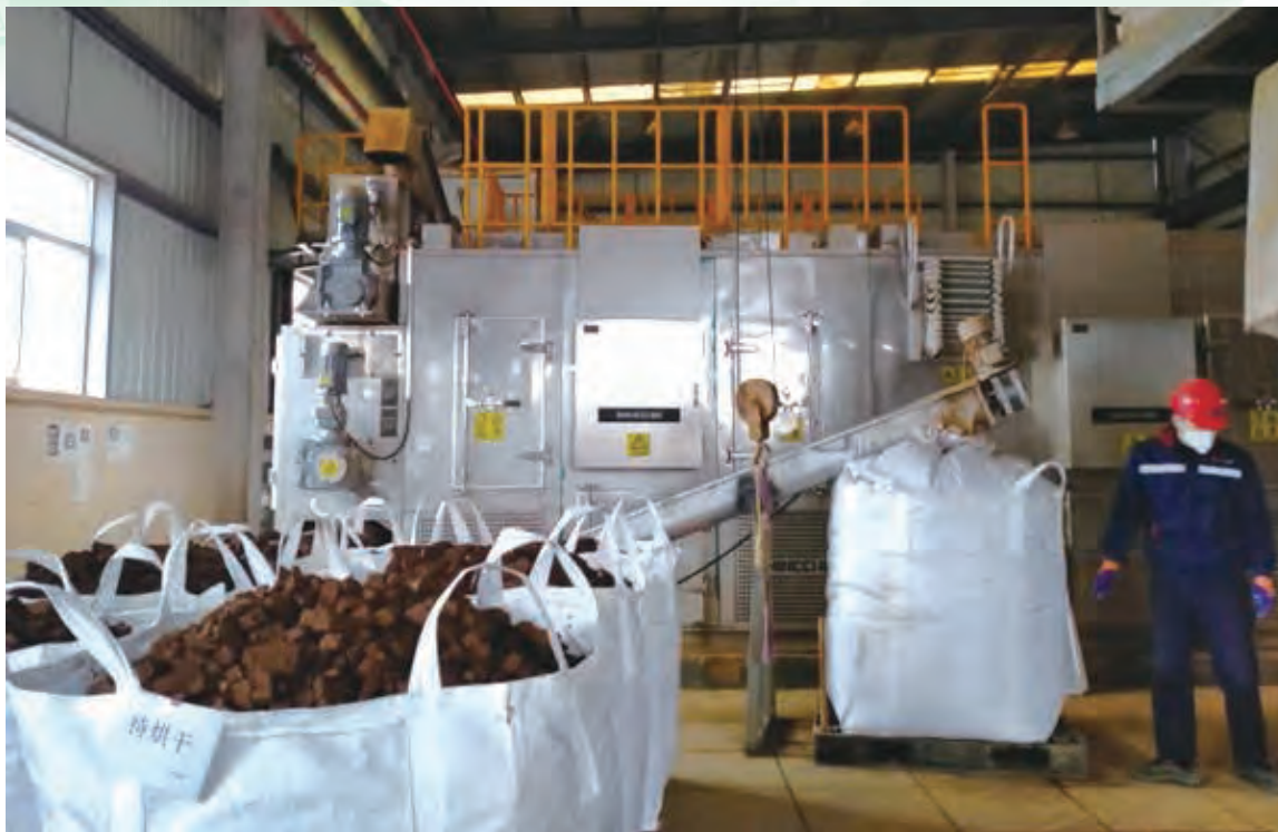
Figure 5 Low-temperature sludge dehydration equipment at Zhenjiang Sinotech
