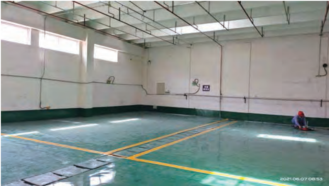
Figure 6 Seepage and leakage prevention work at waste treatment facility located at Yancheng NUHF 圖6 鹽城新宇輝豐廢水處理設施防滲防漏工作
