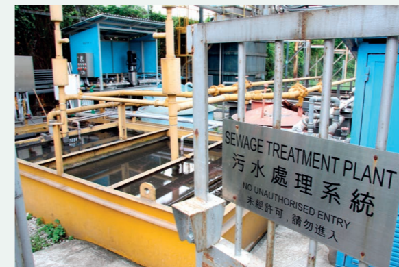
Alliance Construction Material's sewage treatment plant.
