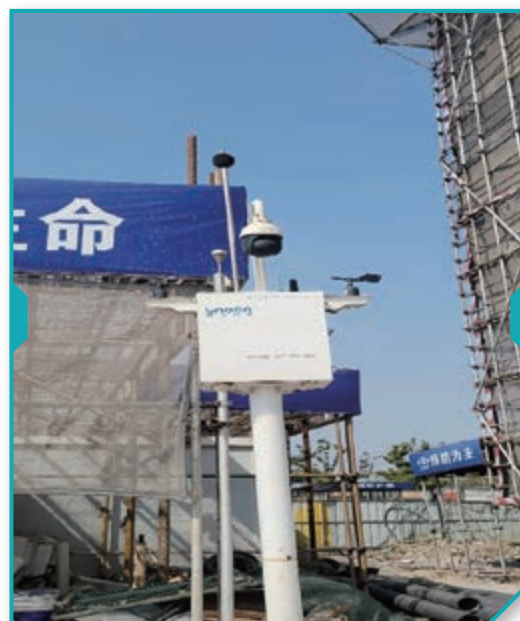
Noise dosimeters are installed at construction site to monitor noise level. Meter reading is recorded few times a day at random intervals serving as random inspections.
