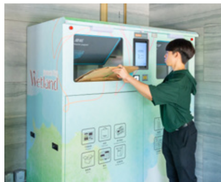
Wetland Seasons Bay's residents can earn points by reducing and recycling waste using smart recycling machine
