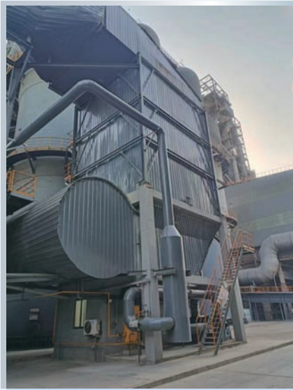
#1 2,000 m 3 blast furnace hot blast stove denitrification 1號2,000立方米高爐熱風爐脫硝
