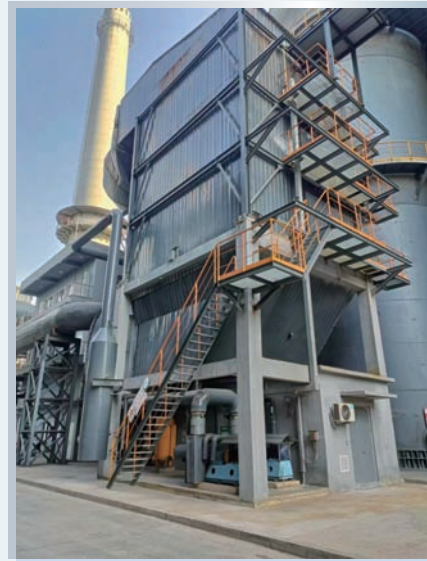
#2 2,000 m 3 blast furnace hot blast stove denitrification 2號2,000立方米高爐熱風爐脫硝
