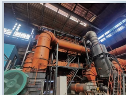
Section steel plant heating furnace denitrification 型鋼廠加熱爐脫硝
