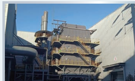
Sheet piling line heating furnace denitrification 鋼板樁線加熱爐脫硝
