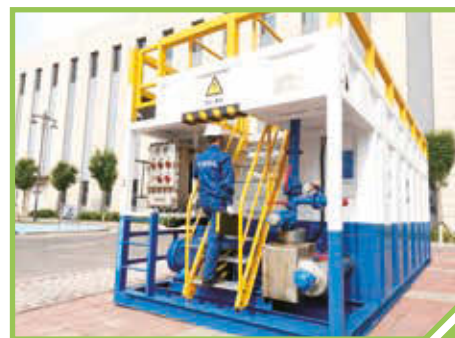
In 2022, 11 inclined ladders of mixed water tanks were rebuilt and put into use at the cementing operation site, so as to reduce the risk of employees falling off when going up and down the water tanks and ensure the safety of operators.
