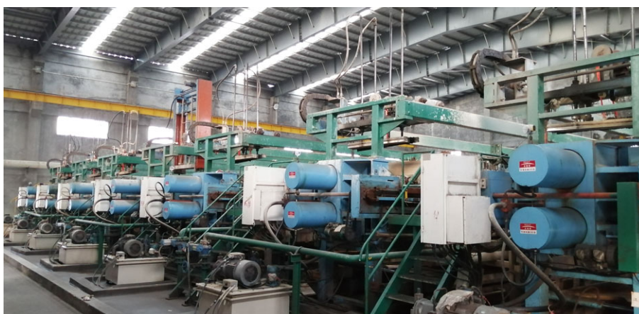
Sludge recycling equipment 污泥回收設備
