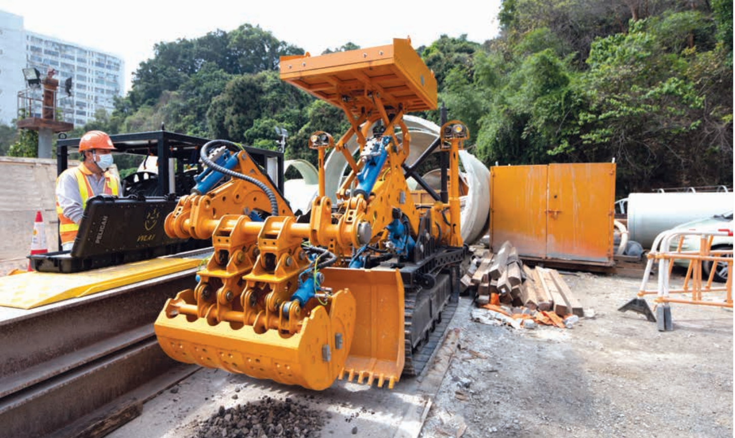
Rehabilitation of Trunk Sewers in Tuen Mun 屯門污水幹渠修復工程
