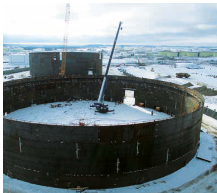
Expanding capacity through assets such as this oil tank at the Hardisty Terminal ensures stable long-term revenues for HMLP.
