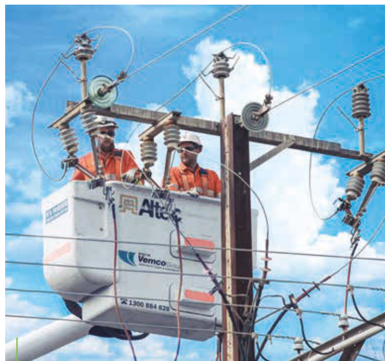
SAPN technicians carry out work on overhead power lines to maintain safety standards.
