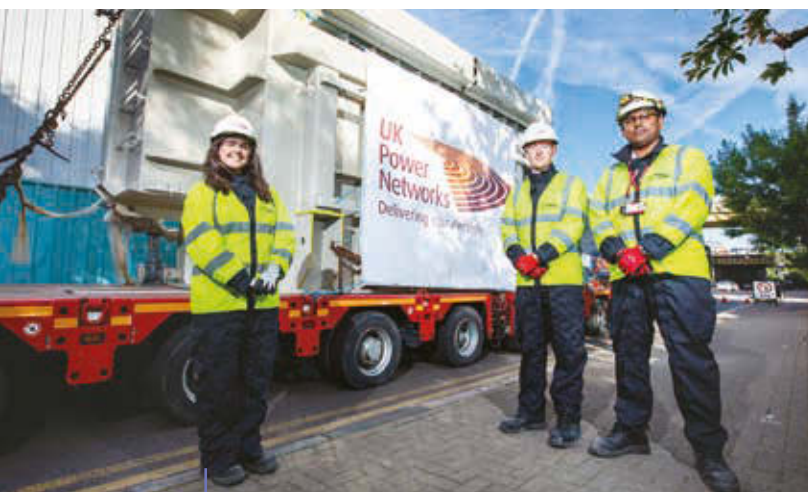
UKPN makes progress on major infrastructure upgrades in London, as part of the ED1SON Alliance, while safeguarding employees.
