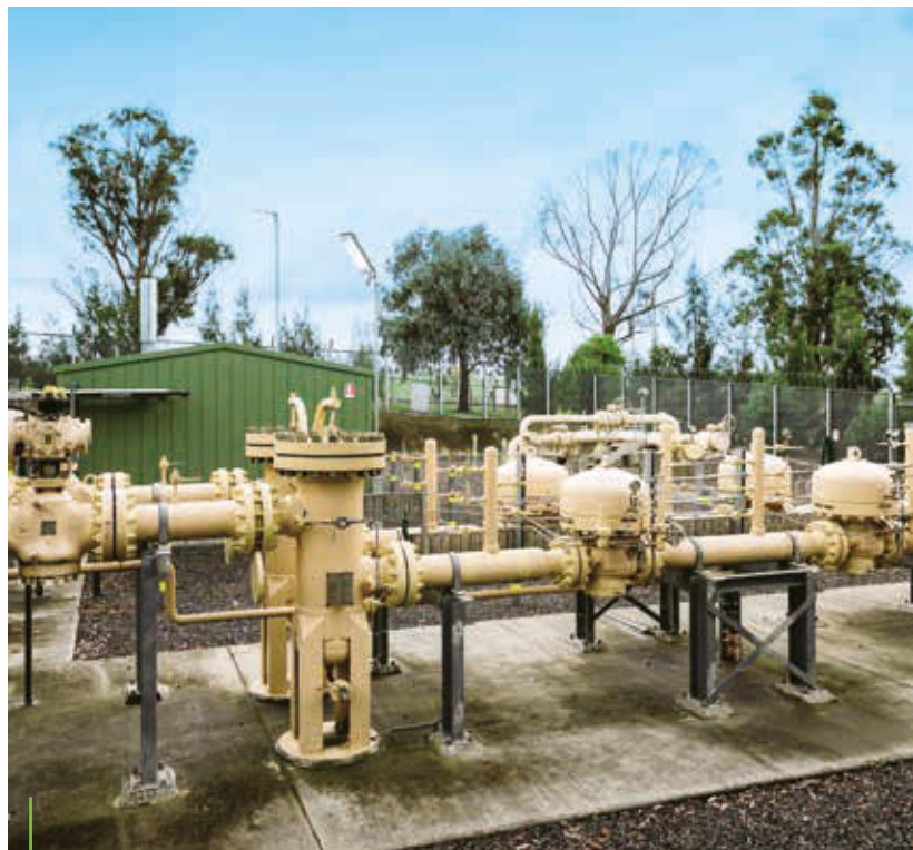
The MG pipeline network distributes natural gas to over 700,000 customers in the eastern and south-eastern suburbs of Melbourne.
