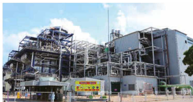
RPCL's power plant exceeds performance and operational targets, securing incentive payments from the government.
