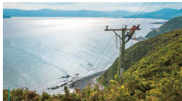
WELL remains committed to investing in its infrastructure such as the refurbishment of power lines at Golans Valley, Wainuiomata.
