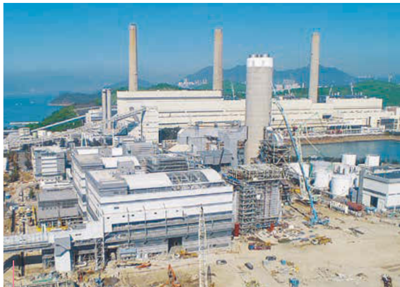
HK Electric's Lamma Power Station progresses well with its development programme. Two more gas-fired units are being built following the commissioning of L10 in 2020.
