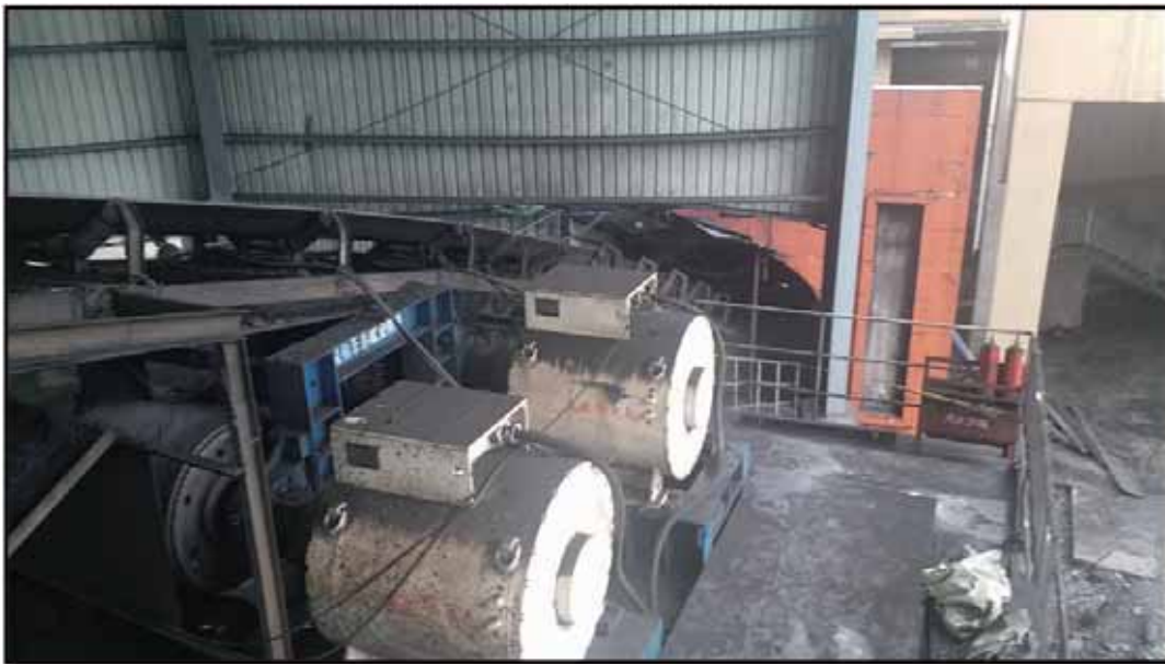
Figure 9-5: Main Decline installed with the main conveyor of the Xiejiahegou Underground Coal Mine
